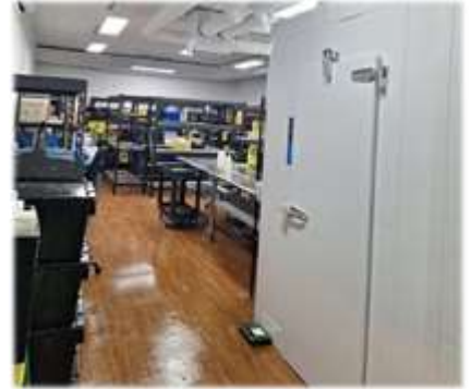
New walk-in fridge and freezer
