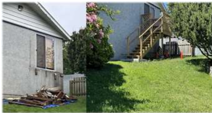
Before and after of the deck and stairs repair at South Island Centre
